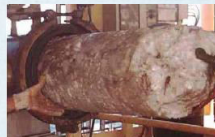
Fig. 3. methane hydrate formation in oil pipeline http://www.rschem.com/solutions/flow-assurance-services
